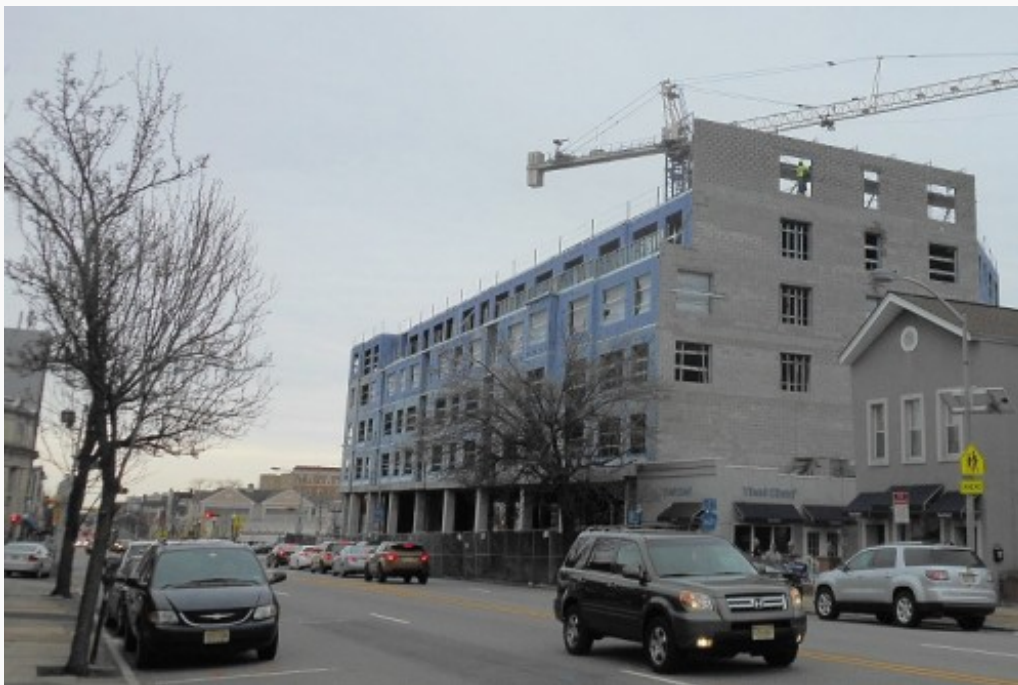
The larger of the two Valley & Bloom apartment buildings, called Building 2, under construction, photographed on April 8, 2015. The topping-out is expected soon.
